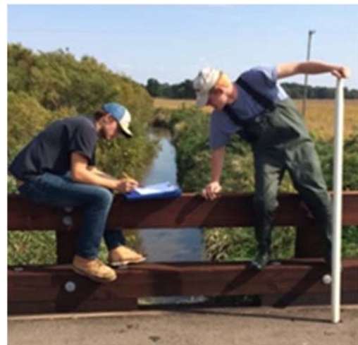
Pictured to the left, is a road/stream crossing located on Rice Creek. This particular crossing is severely undersized. The high velocity shown at the inlet and the restrictive size in relation to bankfull width upstream makes this site a priority for replacement. Pictured to the right, are two of our volunteers. Logan Kreiger (left) and Cullen Hielser (right). Both were being trained on correctly recording data and taking measurements.
